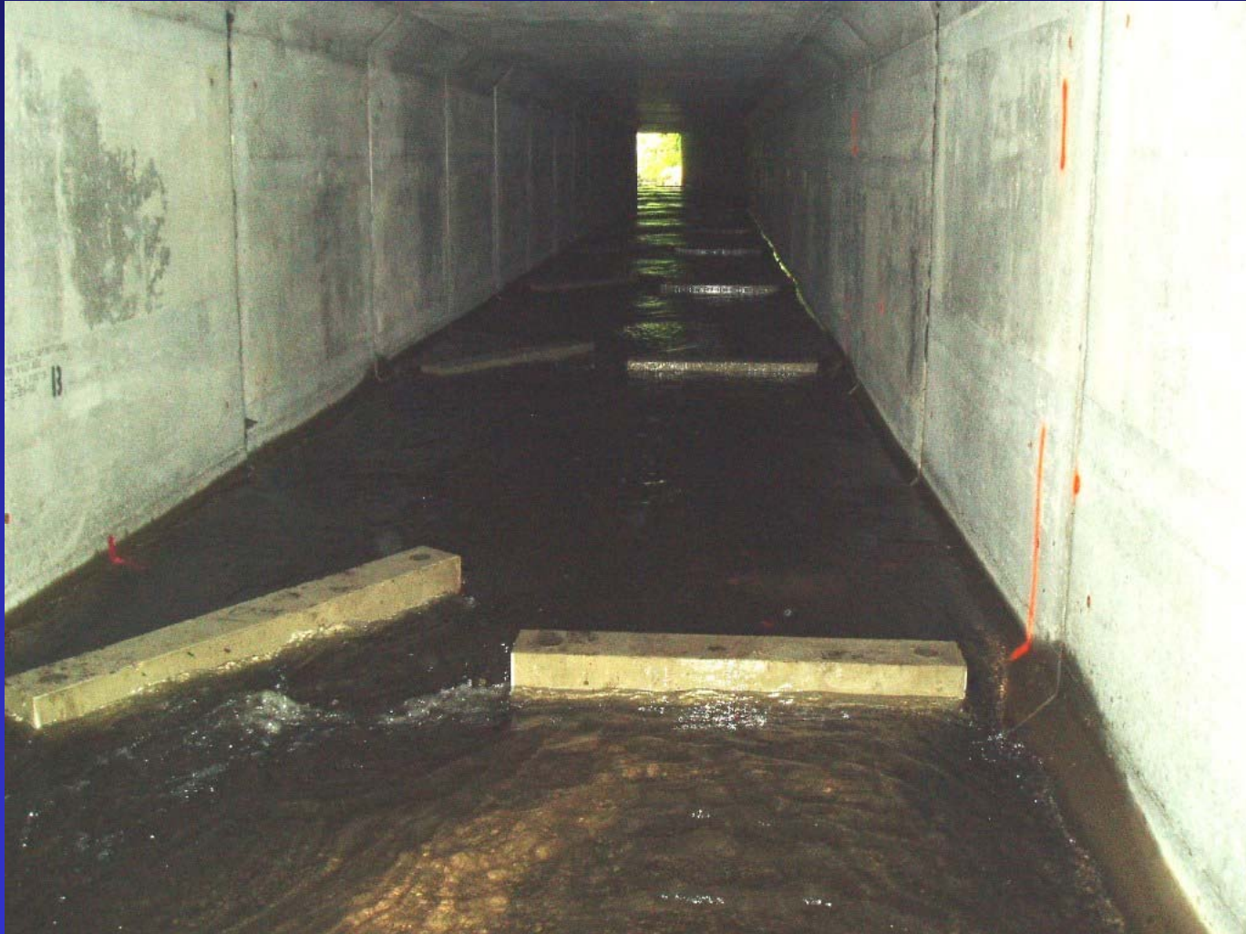
Off-set baffles installed within a box culvert
